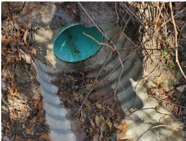
Figure 2-1: PVC Pipe Outlet into the CSV Half-Pipe
