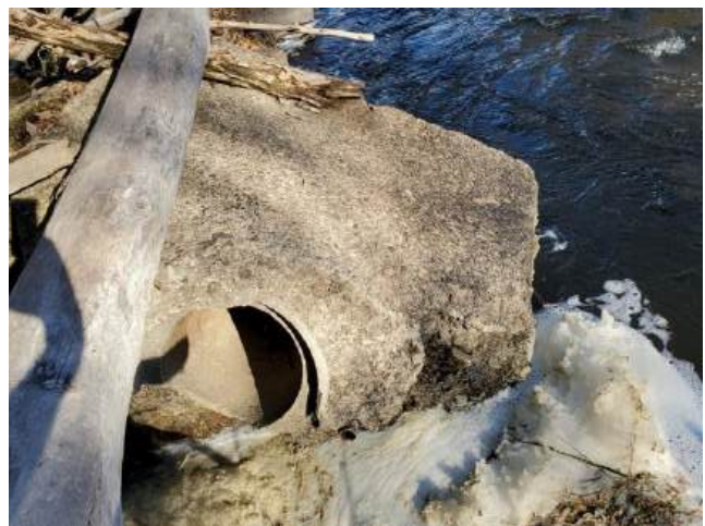
Figure 2-2: Failed Concrete Headwall and Pipe Segment
