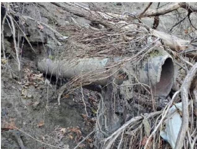
Figure 2-3: Remaining Pipe Protruding from the Slope
