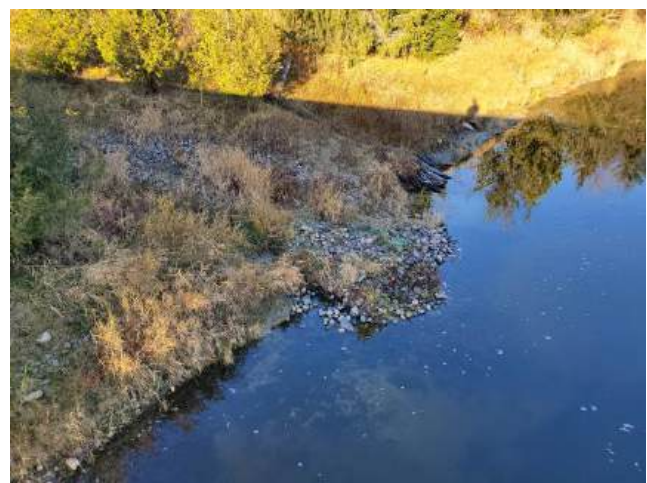
Figure 2-4: Washed Out Swale
