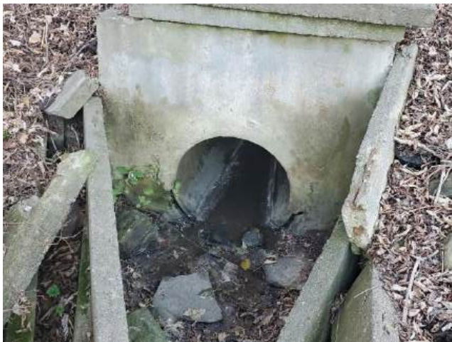
Figure 2-1: Concrete Pipe Outlet with Headwall and Failed Wingwalls
