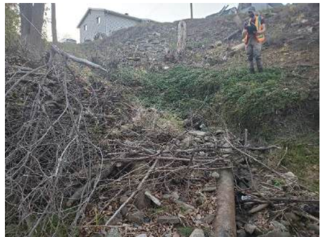
Figure 2-4: Erosion at the Downstream Extents of the Outfall Channel (Looking Upstream)
