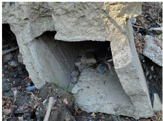
Figure 2-4: Possible Rubble from a Failed Manhole
