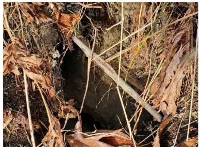
Figure 2-4: Scouring at Recessed Concrete Pipe Outlet
