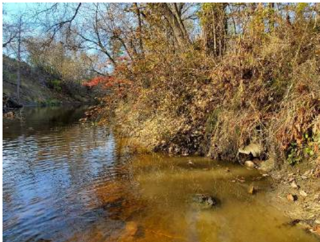
Figure 2-1: Detached Concrete Pipe Segment
