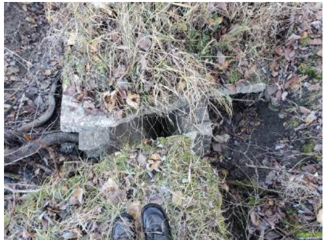
Figure 2-2: Failed Box Culvert (Box Culvert #2)
