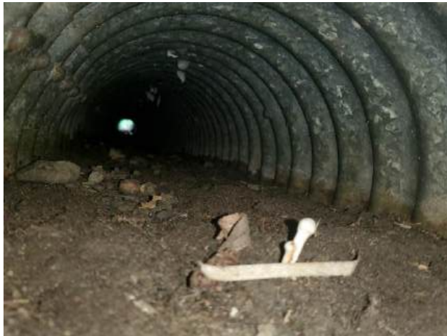
Figure 2-3: Sediment Deposits Inside the CSP
