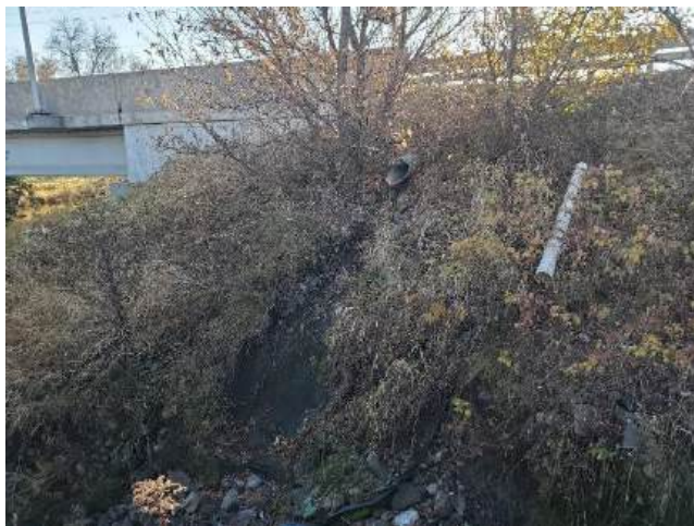
Figure 2-1: Outlet and Eroded Bank
