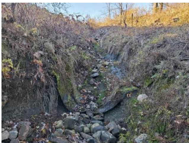
Figure 2-3: Bank Erosion and Exposed Geotextile
