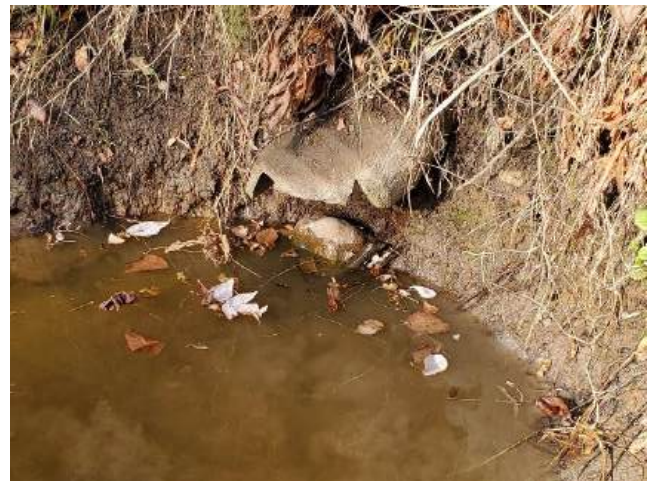
Figure 2-2: Close-up Photo of the Detached Concrete Pipe Segment
