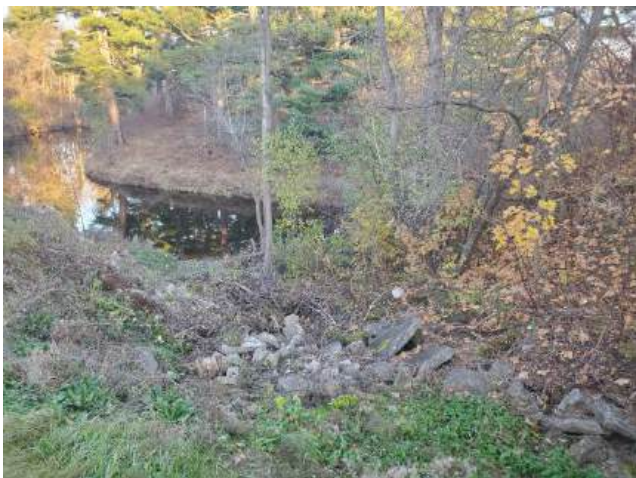
Figure 2-3: Erosion at the Downstream Extents of the Outfall Channel (Looking Downstream)
