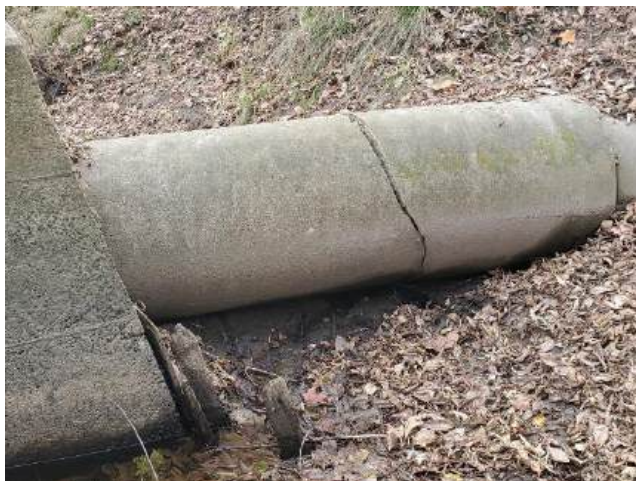
Figure 2-3: Cracked Concrete Pipe
