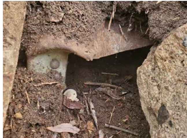
Figure 2-4: Crushed and Recessed CSP Outlet, Surrounded by Concrete Rubble
