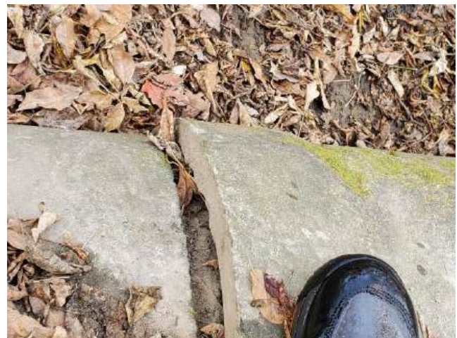
Figure 2-4: Disconnected Pipe Segments
