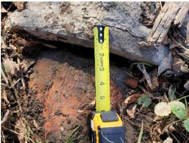
Figure 2-1: Gap Between the Cast Iron and Clay Pipe Segments
