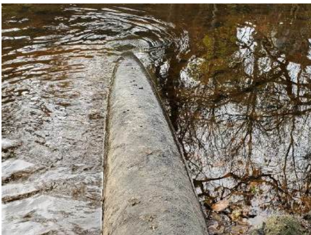
Figure 2-3: Close-up View of the Cast Iron Pipe
