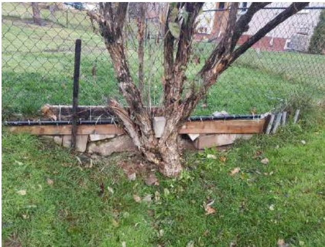
Figure 2-1: Upstream Collapsed Box Culvert
