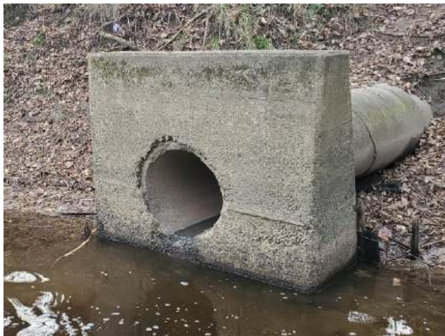
Figure 2-1: Outflanked Outlet Pipe
