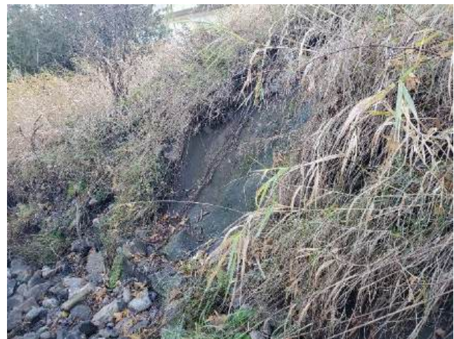
Figure 2-2: Eroded Bank at Outlet
